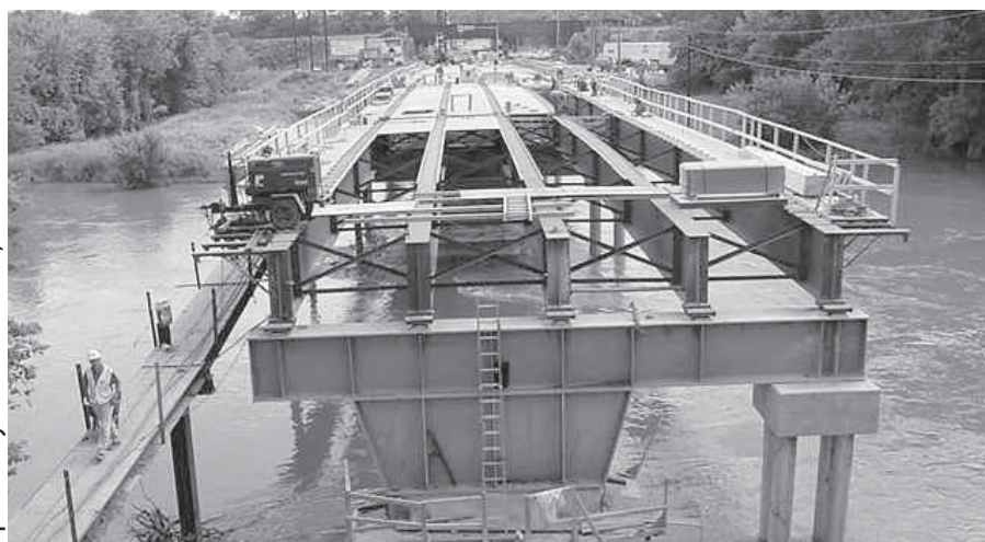
A snapshot from July 12, 2003 of deck work being performed on the award-winning, “Fast Track” U.S. Route 22 bridge in District 6’s Pickaway County.
