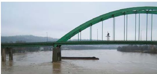
Runaway barges hit the I-70 Fort Henry Bridge spanning the Ohio River between Ohio and West Virginia, outside of Belmont County.
