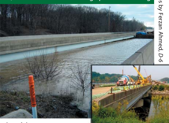
High water flowing under the U.S. Route 36 bridge over Alum Creek in Delaware Co. on Jan. 14, inset with the same bridge prior to flooding.
