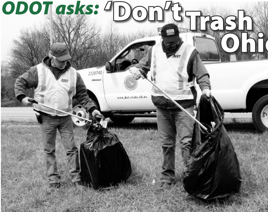
Highway Technician 2s Mike Charlton (left) and Curtis George from ODOT D-6's Westerville Garage pick up trash on Interstate 270 near Columbus.
