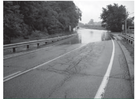
Flooding of State Route 96 at State Route 598 in Crawford County.
