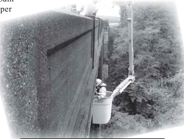
Under-deck truss bridge inspection of the County Route 843-Willard Rd. Bridge in Columbiana County on August 20.
